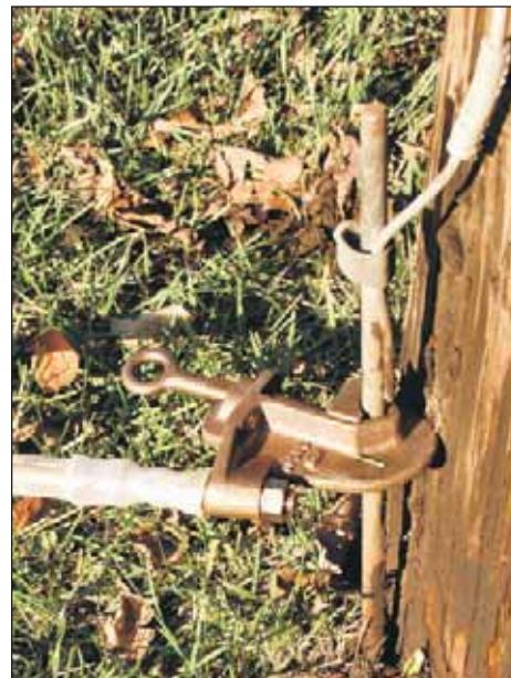
Vertical neutral of a multi-grounded neutral system
